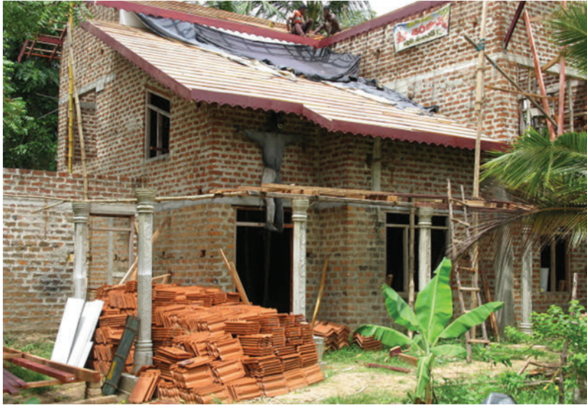
FIGURE 11.4. Walangama two-story house under construction in 2013. Adding a second story increases the number of hierarchical levels in the house's spatial syntax. (Photo: 2013, Deborah Winslow.)
